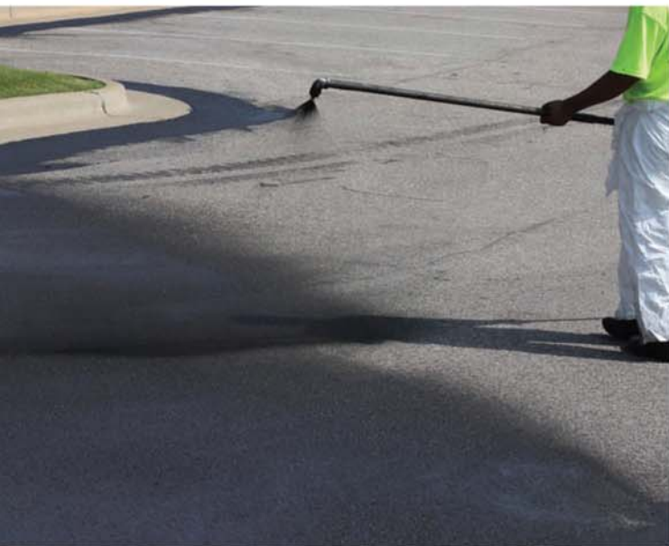
Top: Hand-spreading of sealant using a squeegee should occur in corners, edges and in confined areas.
